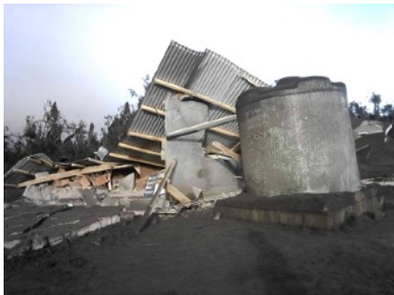
Collapsed church building
