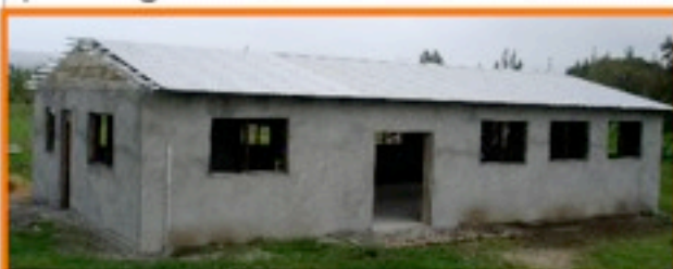
Above: The building now has a roof, but no windows yet. With good weather the building is not far from being finished.
