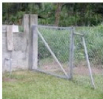
Above: Installing the chain-link fence was completed once we welded and put up a gate.
